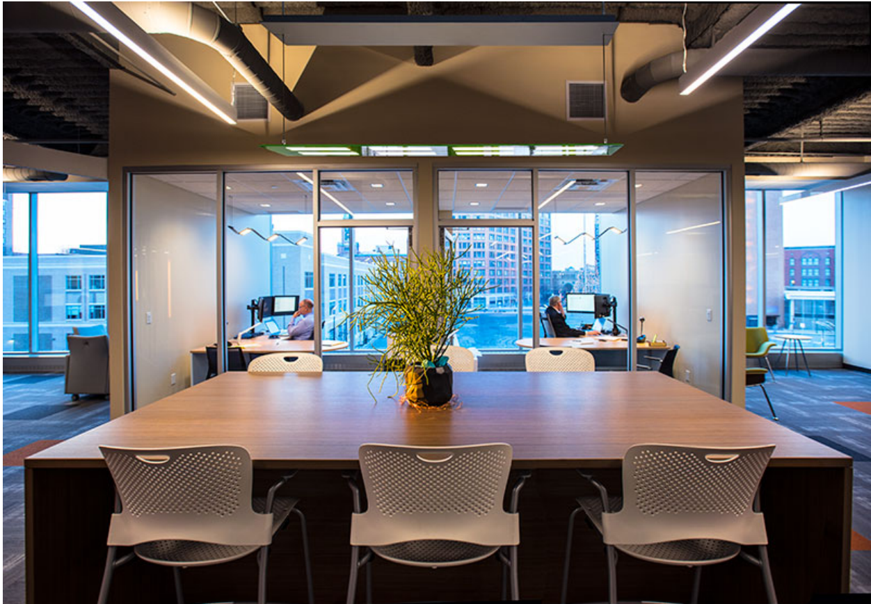
Figure 22. The newly installed Acuity Brands Peerless Olessence™ luminaire, mounted in place of linear LED luminaires in the open office area. Photo courtesy OLEDWorks LLC and DeJoy Knauf & Blood, LLP.
